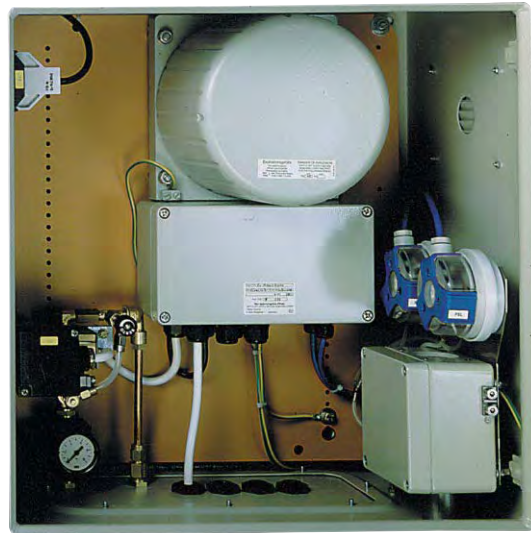
Air Purged Control Panel
